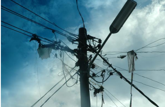
Electrical network in Mozambique. By Mauro Pinto
